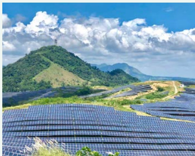
EPI Subic solar panels
