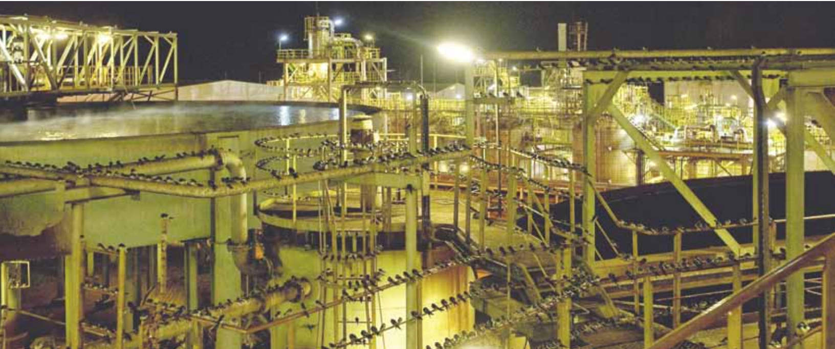
Coral Bay HPAL Plant
